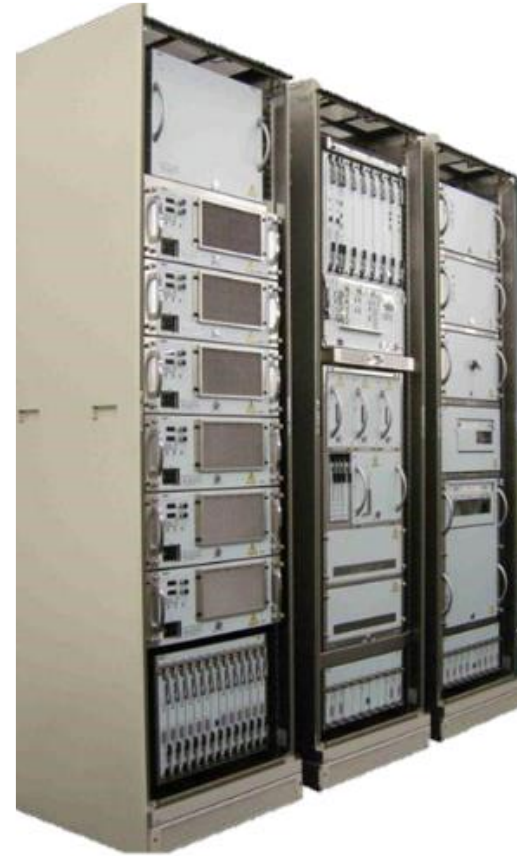
PFE (Power feeding equipment)
